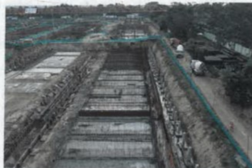
CWSS 5th stage 3 mtr. dia Transmission
